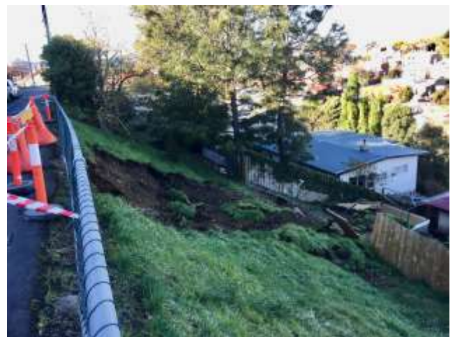
Destruction from landslides downslope from Liverpool Street after rainfall event in 2018 (Photo P. McGoldrick)
