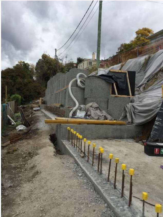
Large concrete blocks forming the wall with concrete poured in between to stabilise the slope beneath Liverpool Street (Photo HCC).
